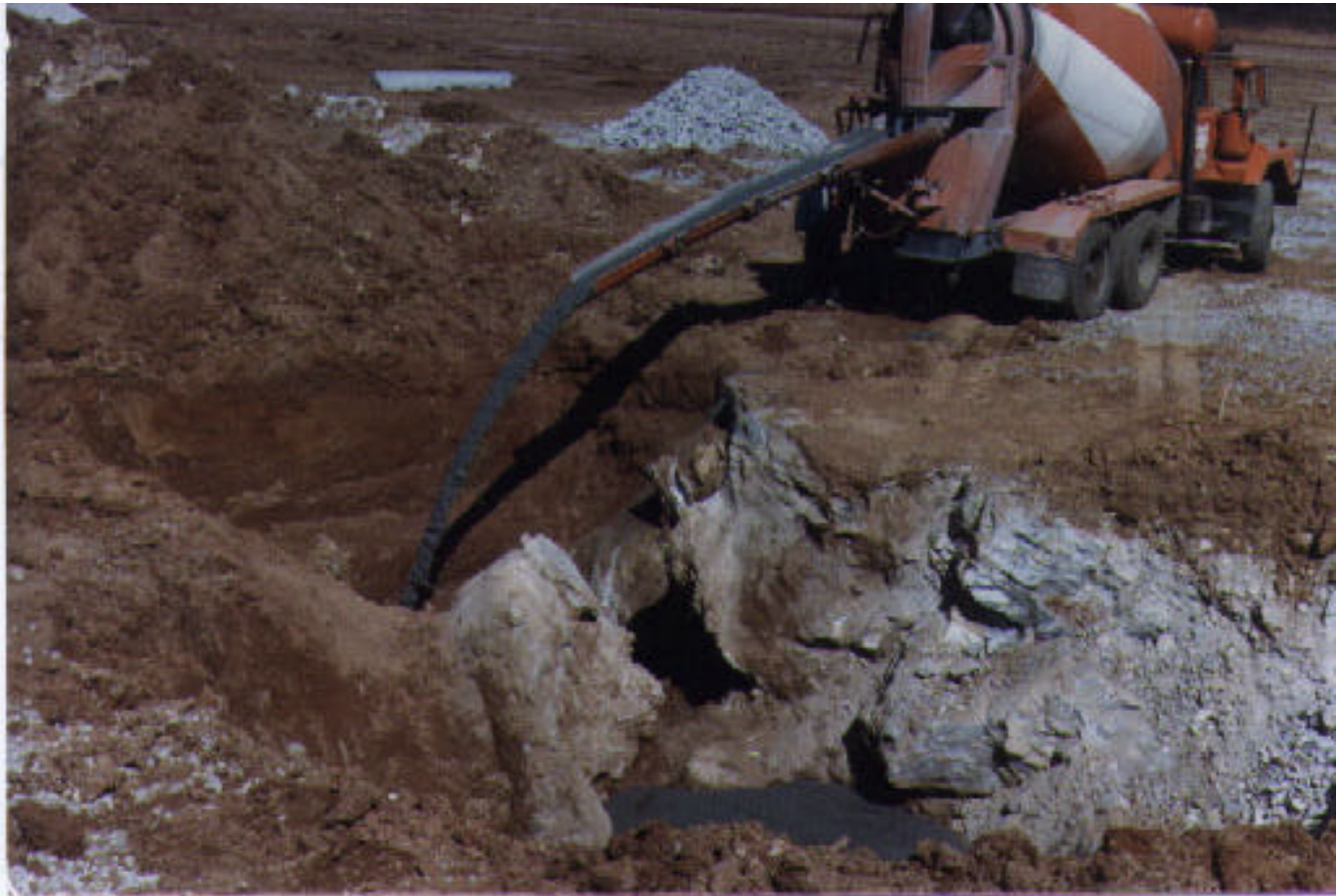
Fig. 4 – Placing grout to seal off the throat of a sinkhole exposed by dynamic compaction
